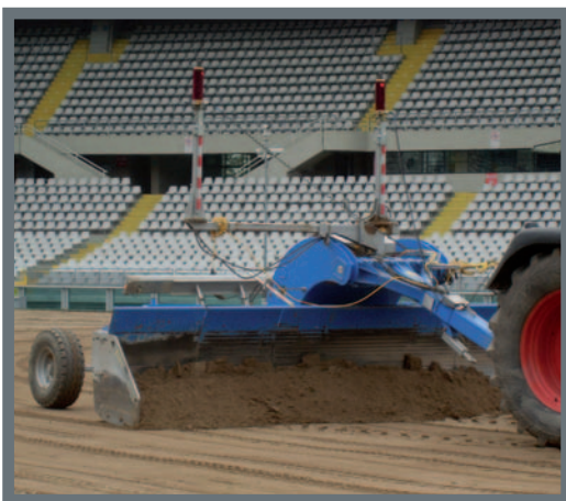
» Stadio delle Alpi — MOBA Dual-Laser-matic used for leveling works in the soccer stadium of AC Turin (Italy)
